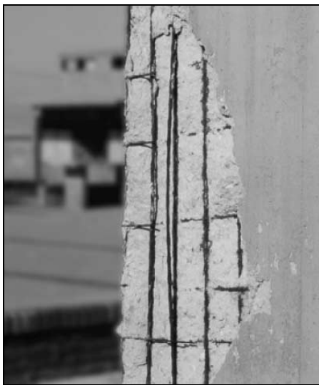
Figure 2 Building 3 —showing that the bars are no longer in contact with the concrete
