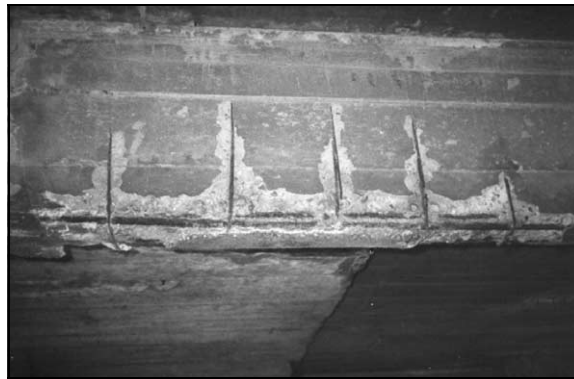
Figure 1 Building 1 —showing spalling and loss in steel section
