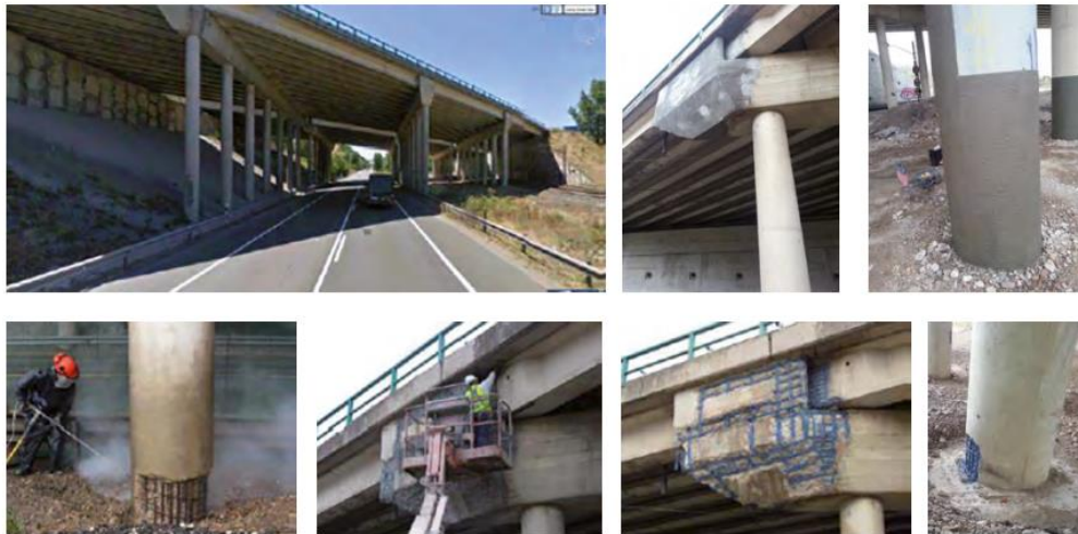
Figure 5. Viaduct on motorway AP-I (Spain) patch-repaired. 3
